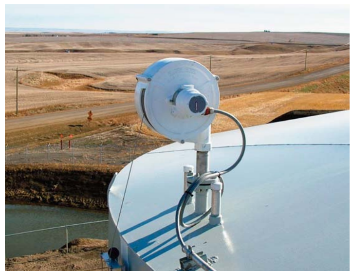
Below: Redtail with Optional Goshawk Transmitter installed on a tank.
